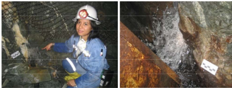
Figure 9 Groundwater inflows through fractures to the tunnel (see online version for colours)
