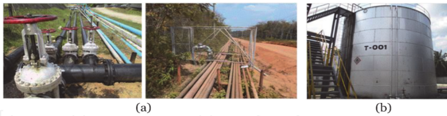
Figure 1. Pipeline system and storage tank for oil gathering activity. (a) Pipeline System. (b) Storage Tank.
