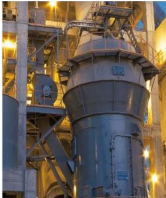
Gambar 2. Vertical Roller Mill Tampak Depan (sumber : PT. Semen Indonesia, 2021)
