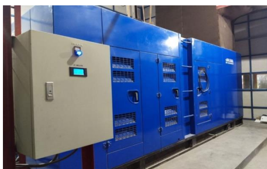
Gambar I.27 Generator Diesel PT.Sinar Sakti Kimia
