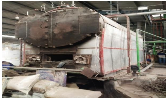
Gambar I.29 Boiler PT. Sinar Sakti Kimia
