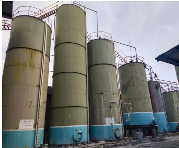
Gambar I.14 Storage Tank PT. Sinar Sakti Kimia
