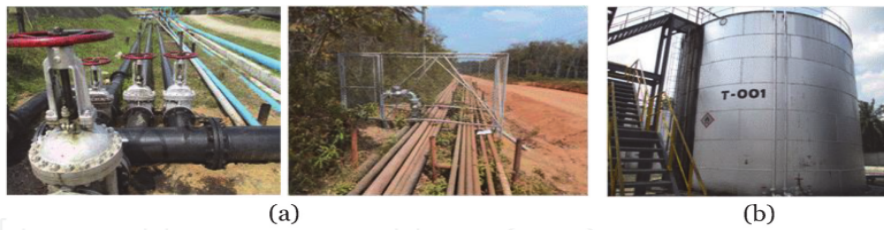
Figure 1. Pipeline system and storage tank for oil gathering activity. (a) Pipeline System. (b) Storage Tank.
