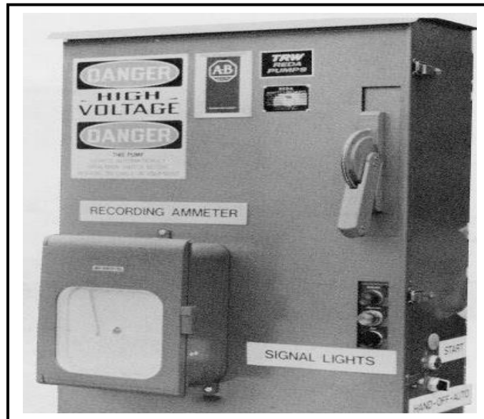
Gambar 3.16. Switchboard (Takacs, Gabor., 2009)
