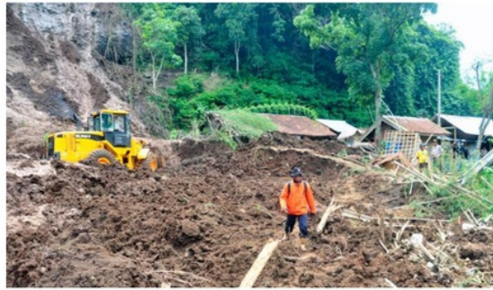
Fig. 6 Landslide of Ngawen, Southern Mountains [13]
