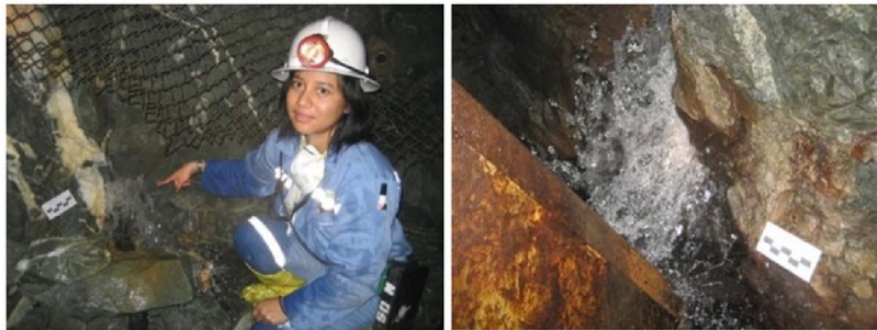
Figure 9 Groundwater inflows through fractures to the tunnel (see online version for colours)
