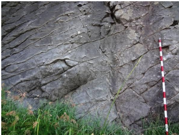
Fig. 13: Sheeting joint at Mt. Lawang
